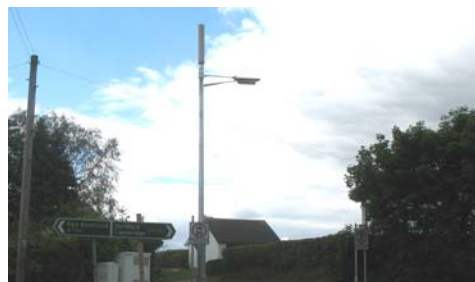
Example of replacement street light incorporating a base station (Source: Agent for T-mobile)
