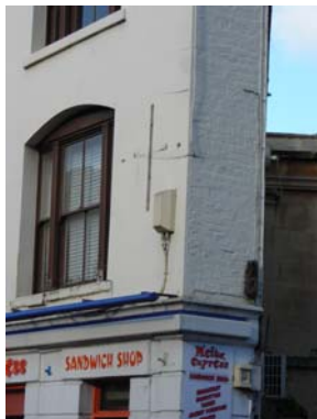
Example of a microcell antenna which could be classed as 'de minimis'
